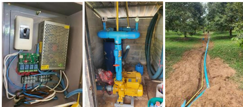
Figure 4. Control unit (A), water pump (B) and test plot and system(C)
